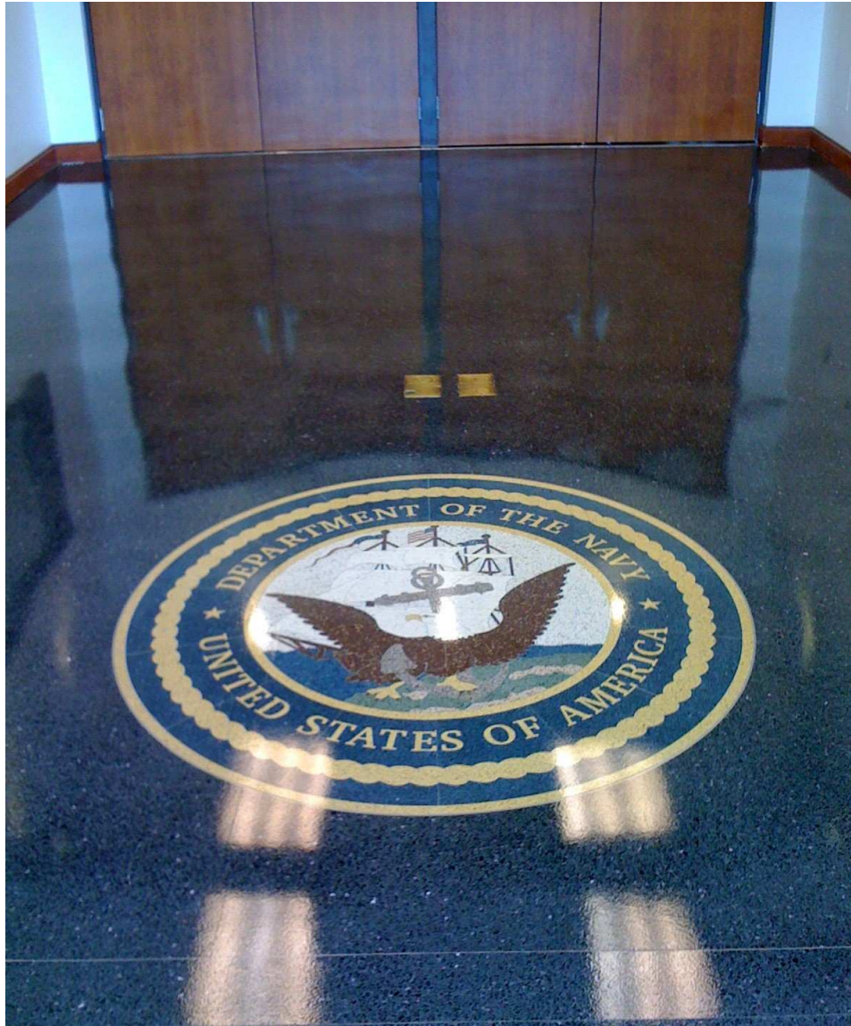
Great Lakes Naval Base - North Chicago, IL The GlossTek Fast Dry was applied on the Terrazzo flooring.
